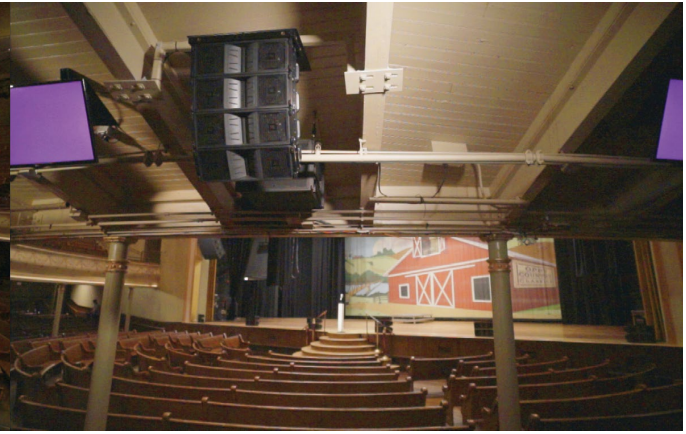
The new under-balcony system includes JBL VT486s with time-aligned VT4883 subwoofers.
